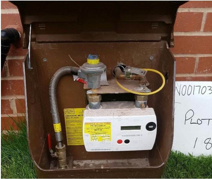
Copper pipework has been drilled through the rear of the multi box and not been put through the purpose built hole in the side of the box.
