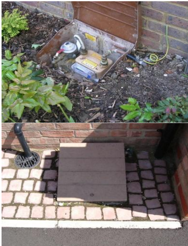
Meter box too low, potential for water ingress, landscaping should not be this high. Should be approximately 50mm below front edge.
