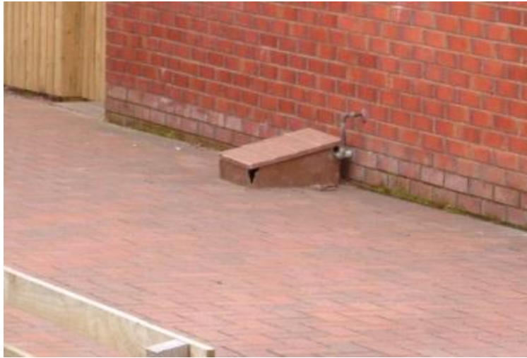
Semi concealed meter box in driveway, not permitted, only recessed meter box fitted into wall as susceptible to vehicular impact.
