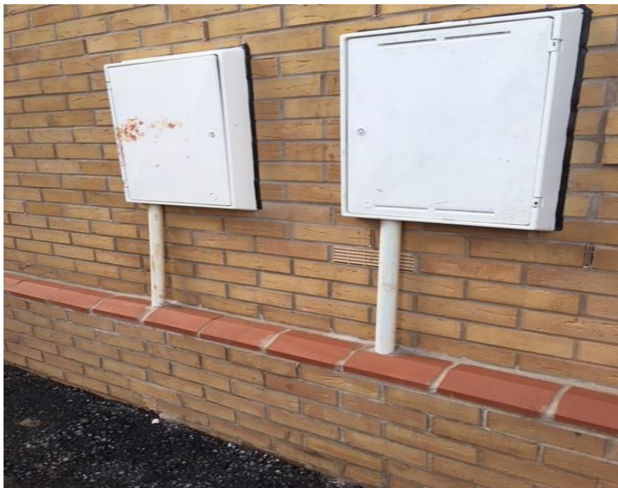
Unapproved method of covering electric hockey stick and gas riser.
