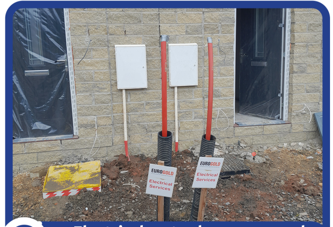
✓ Electrical meter boxes secured and tails labelled.
