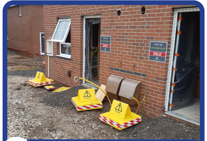
✓ Meter boxes correctly installed.
